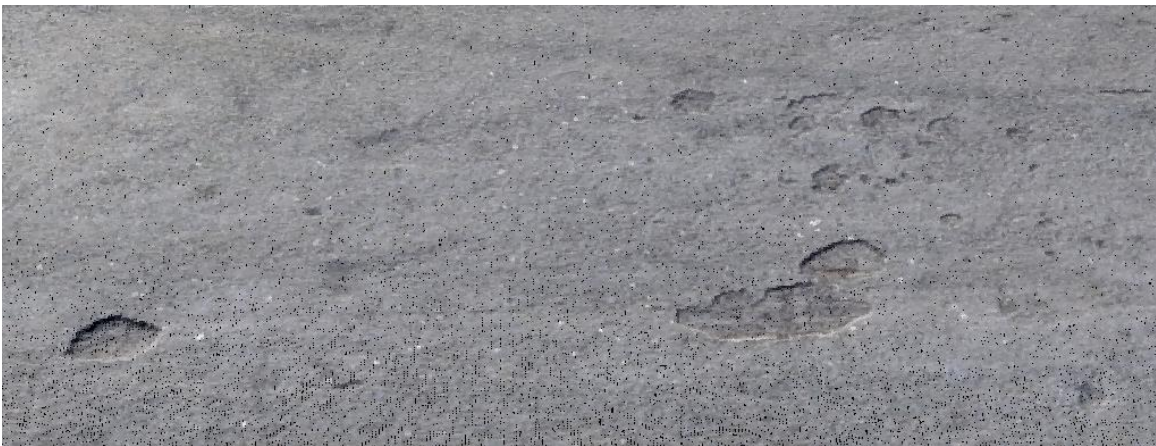
Figure 46. The density of the Pix4D point cloud make it possible to view things like potholes in the parking lot.
